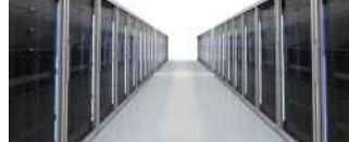
The Toppan Group datacenter (Image is for illustration purposes only.)
