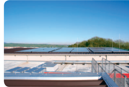
Solar panels on the roof of the factory power the lighting of the administrative offices.
